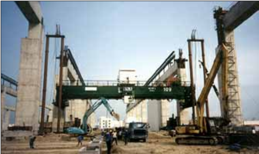
Above and below: the Fagioli PSC designed modular panel tower and lift beam system lifts a 280 tonne crane to the runway beam level.
